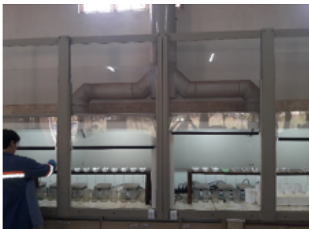
Fig 13 New exhaust system
